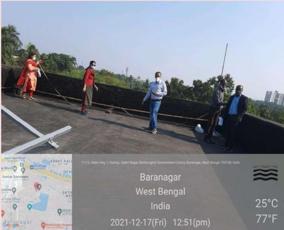
Rain water harvesting measurement (17.12.2021)
