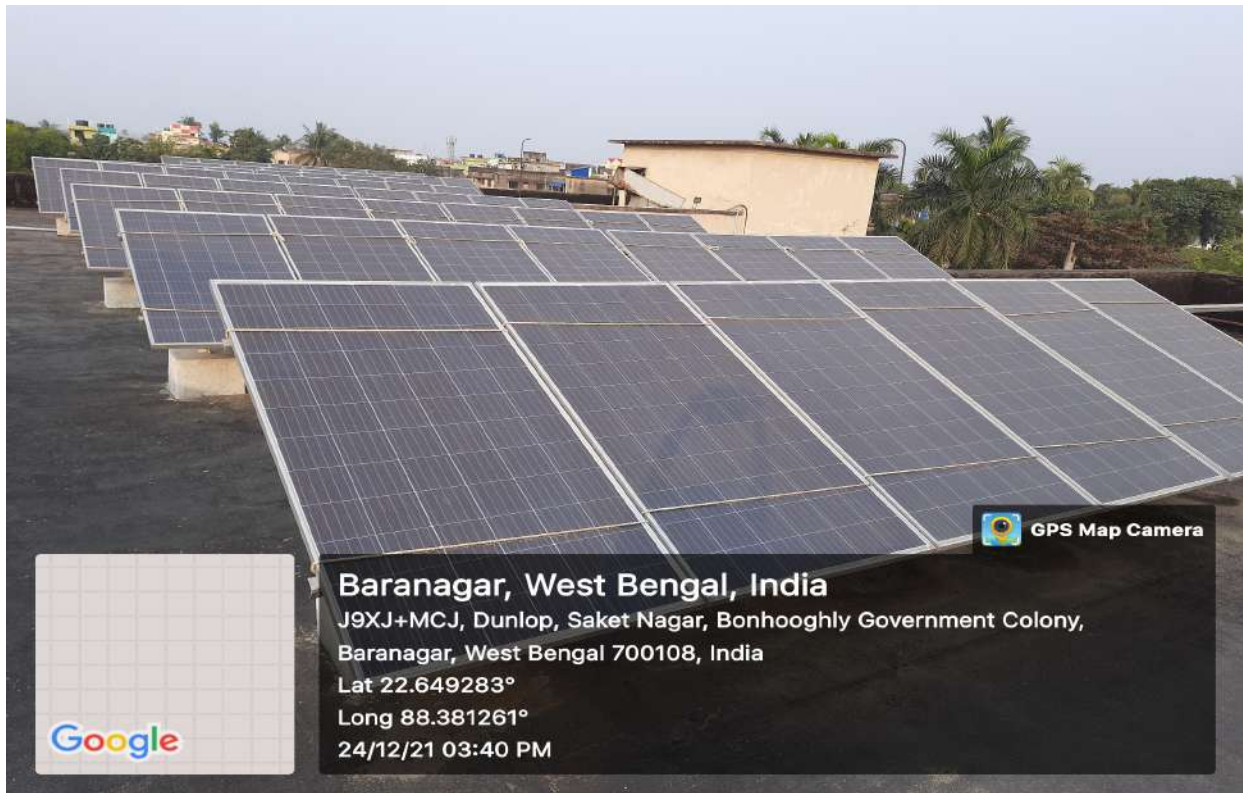
Solar Panels on rooftop
